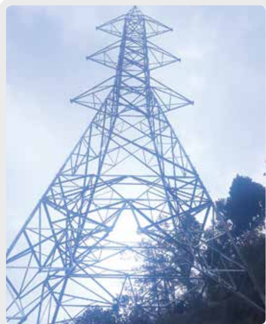
132 kV Transmission Line Tower
