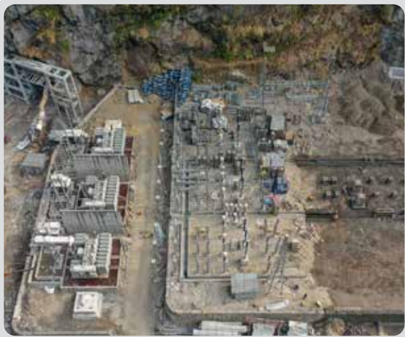
Switchyard Area overview
