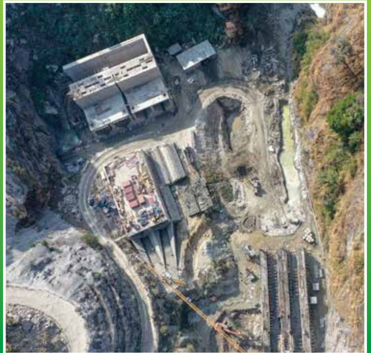
Overall Headwork Overview
