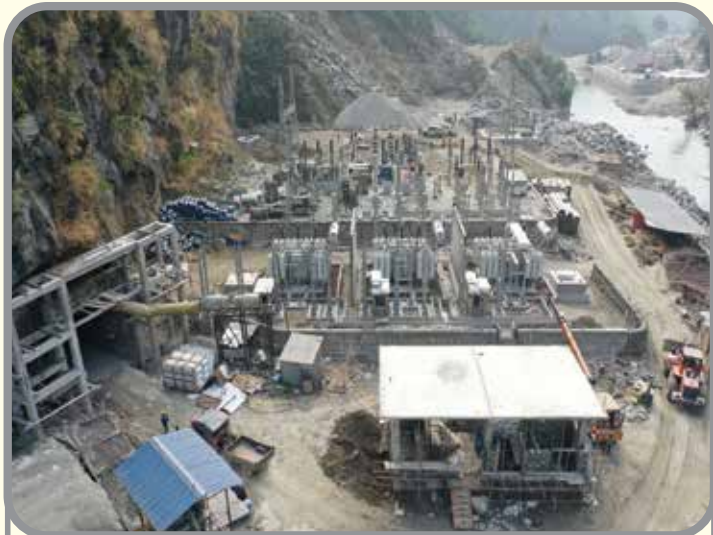
Switchyard Area overview
